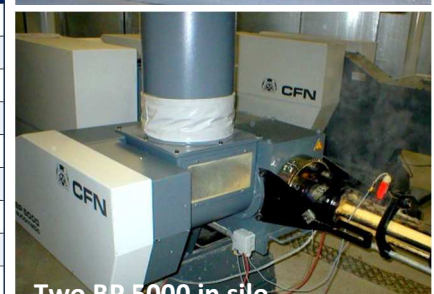
Two BP 5000 in silo
