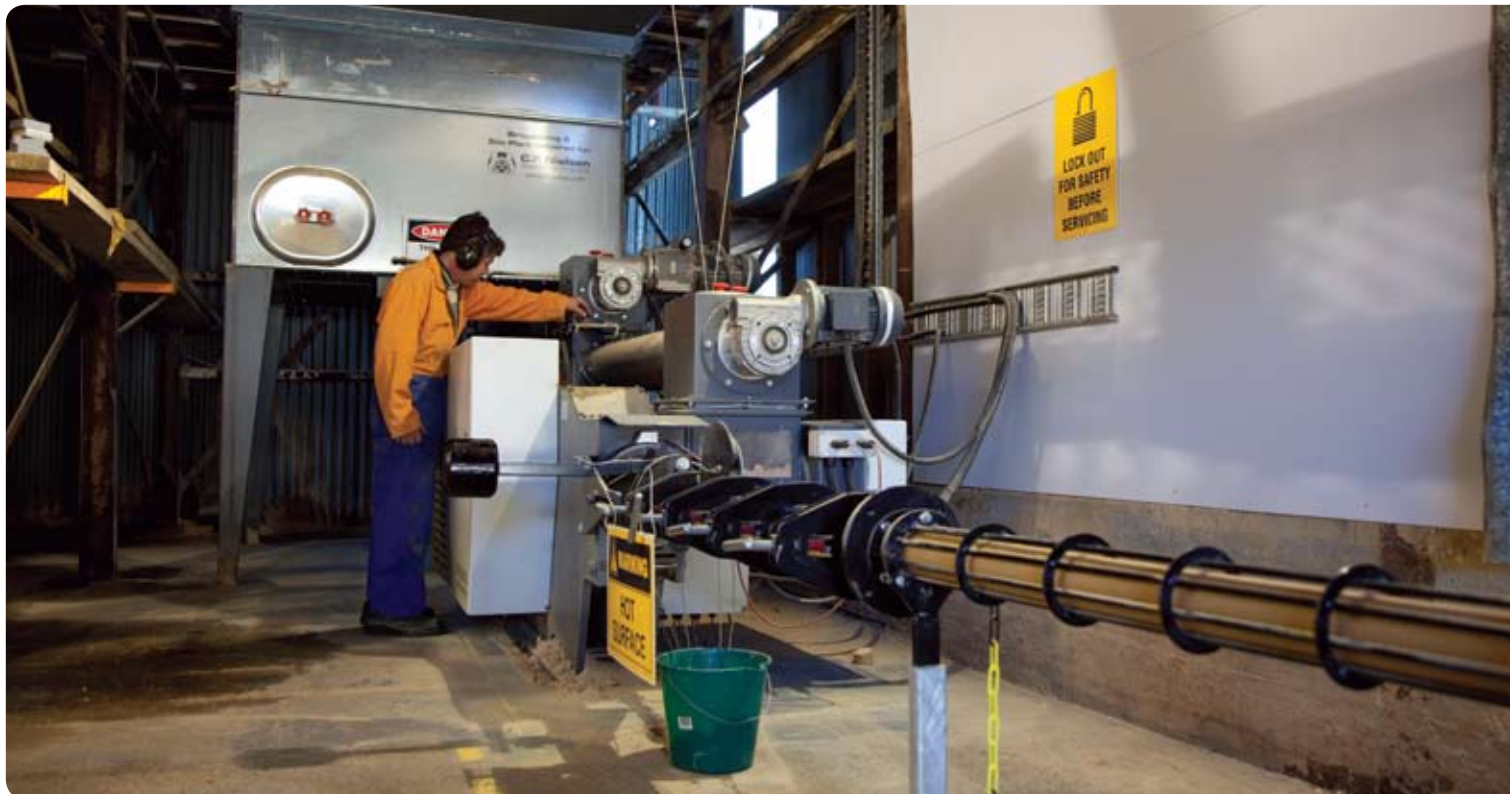
The BP 3200 briquette press, which turns MDF dust into fuel.
